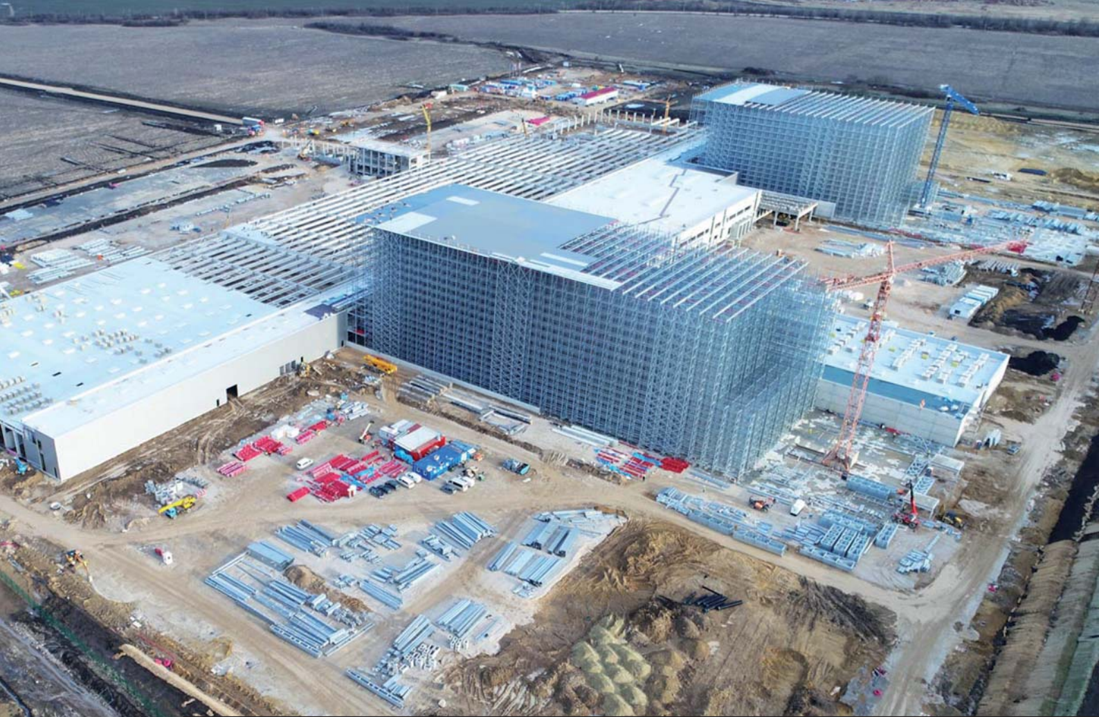
During the construction phase, the gigantic steel skeleton of the high-bay storages was revealed.
