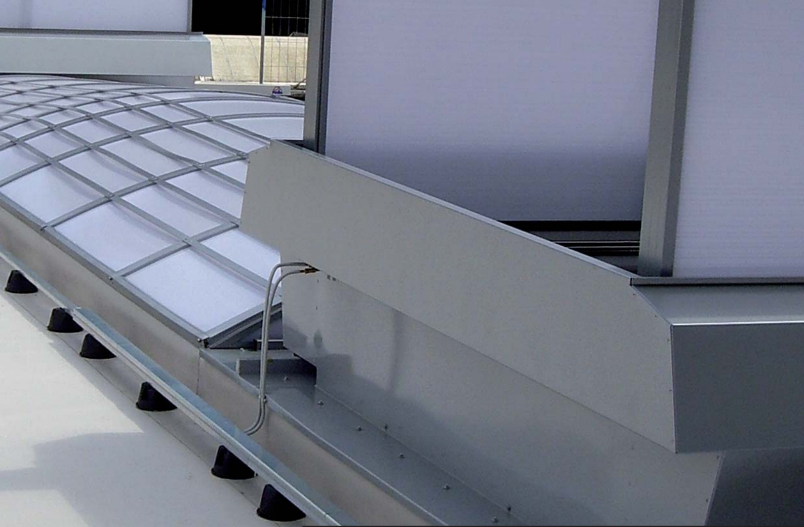
Feeds were led out of the system and laid in cable ducts over the roof.
