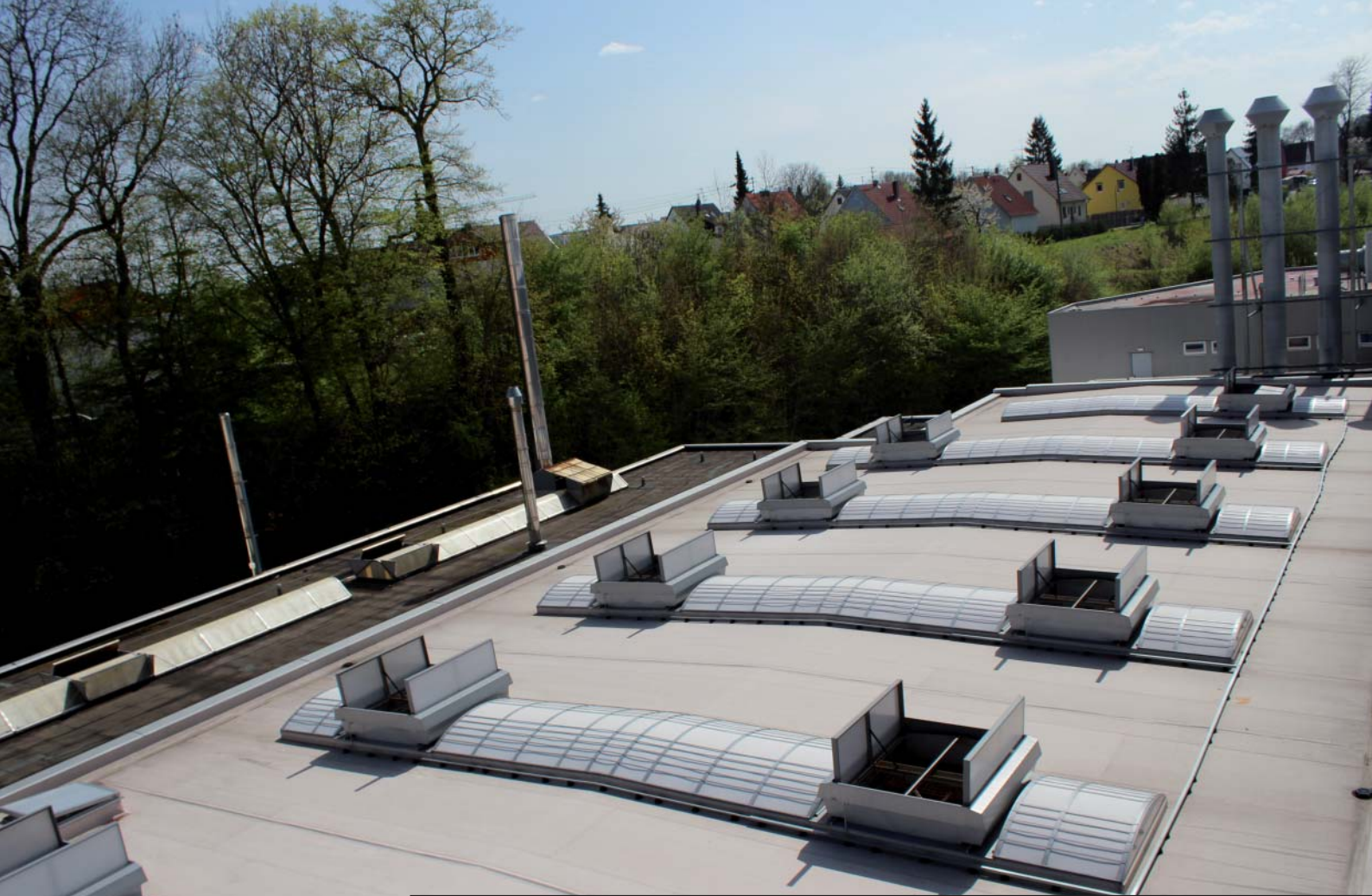
Two MEGAPHOENIX systems were each integrated into one continuous skylight.
