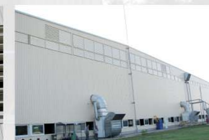
AIRJET mounted in a wall
