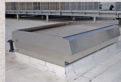
Stand-alone unit on a factory roof
