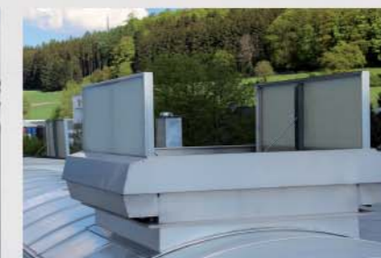
Mounted on an arched skylight
