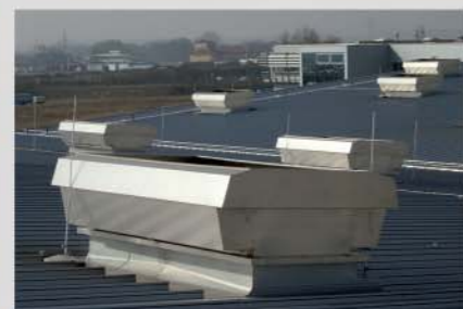
Stand-alone unit on a factory roof
