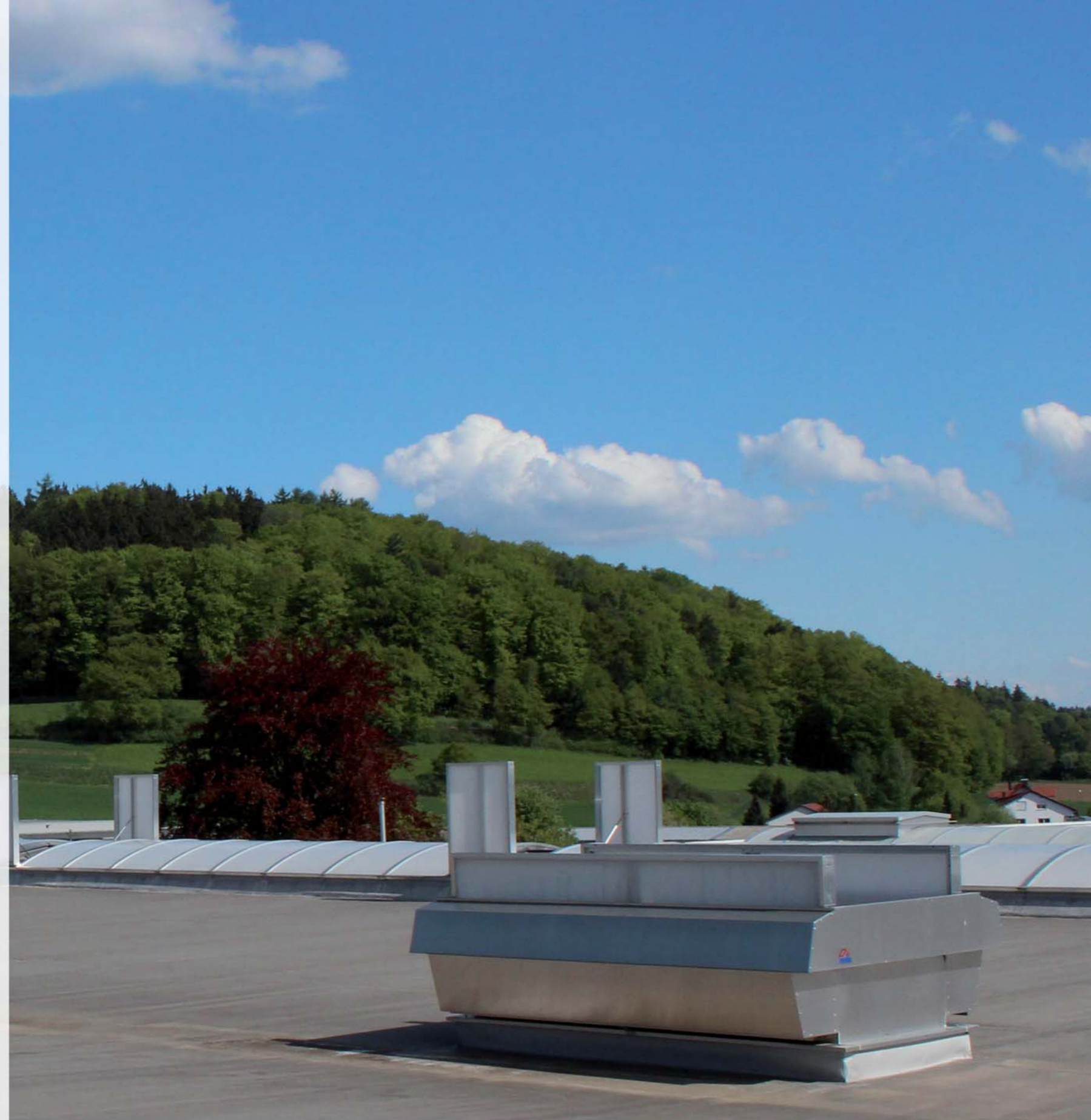
Large illustration: MEGAPHOENIX as a stand-alone unit on a factory roof.
