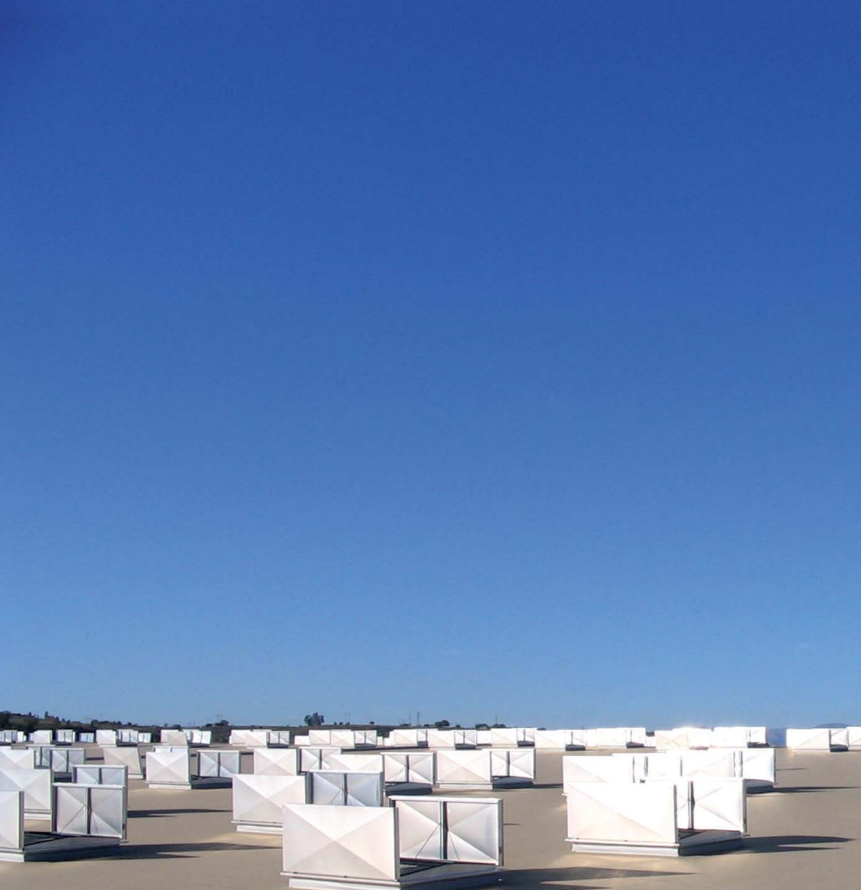
Large illustration: PHOENIX ventilator on a factory roof.
