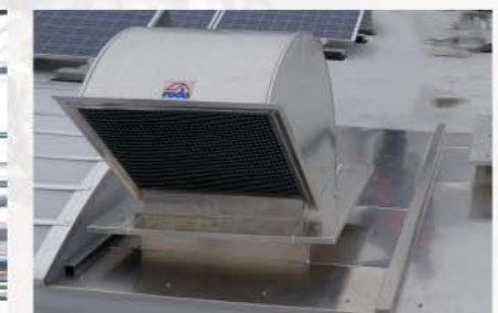
Roof-mounted suction hood
