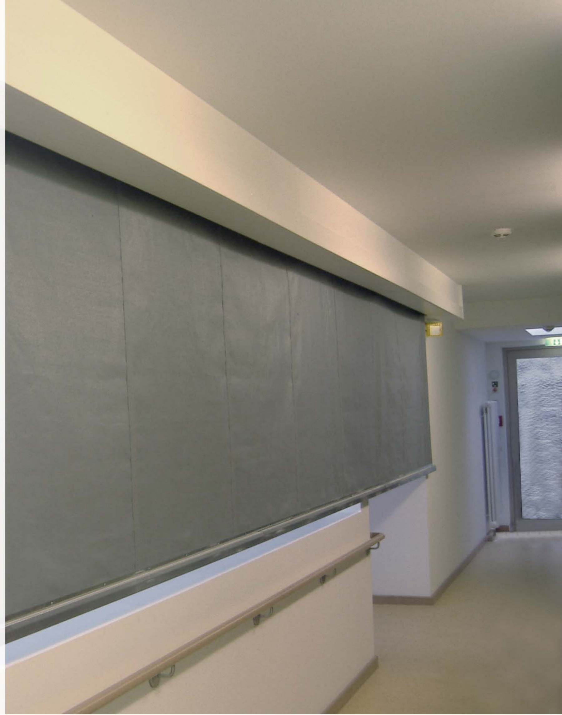
Picture: At the reception desk of this hospital the rolled smoke curtain is visible only when run out in the event of a fire
