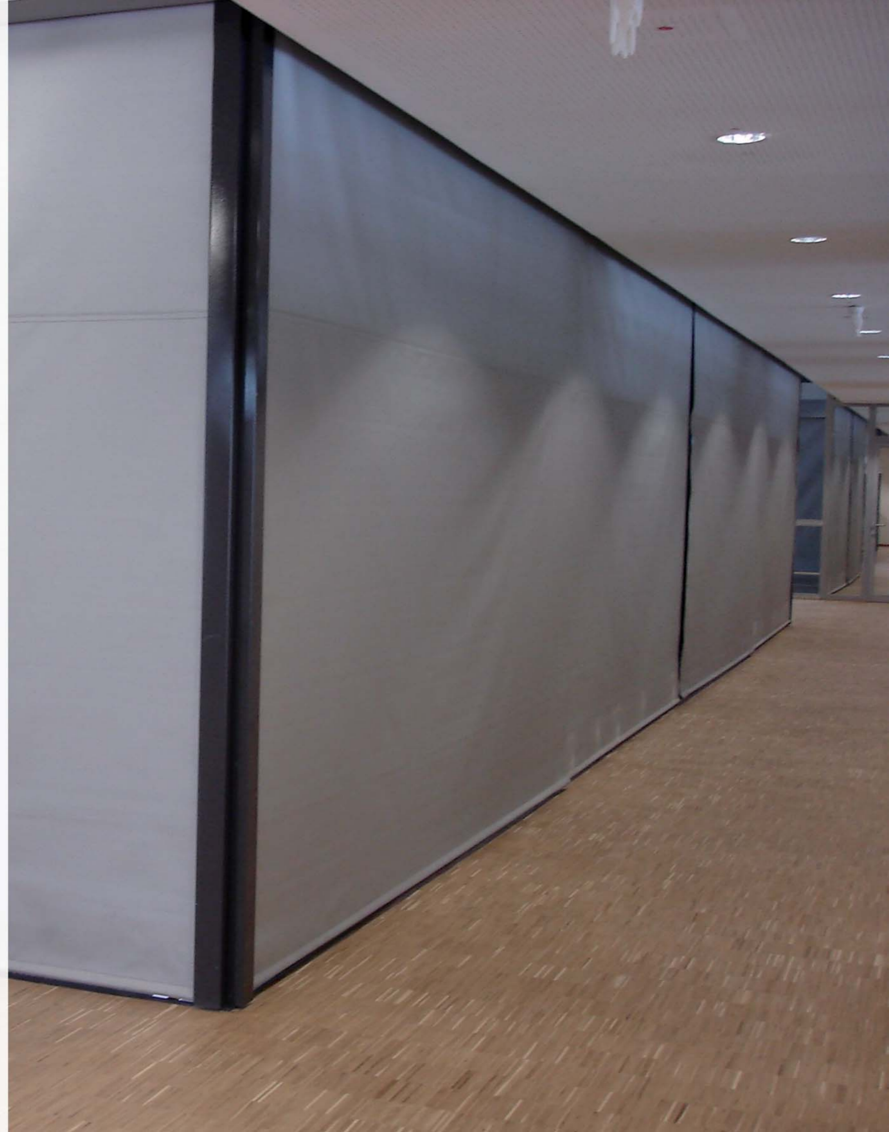
Picture: Smoke curtains keep this floor of a school free of smoke in order to enable people to escape from the building
