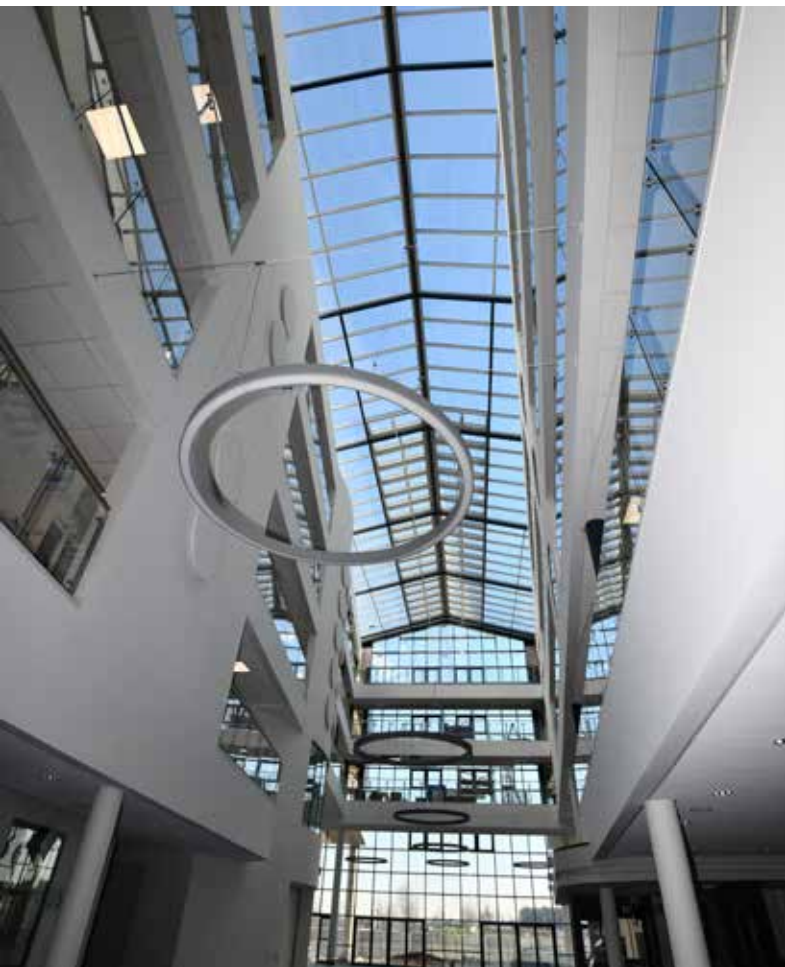
FIREFIGHTER double flap fan installed in a glass roof construction
